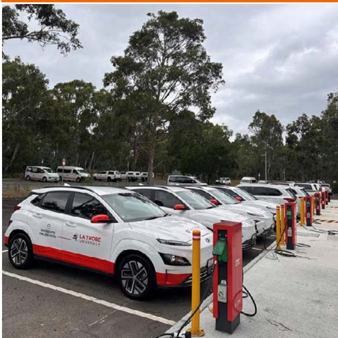
La Trobe University's electric cars being charged at their Bundoora campus
